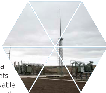
132/22 kV Székesfehérvár South Substation, HU
